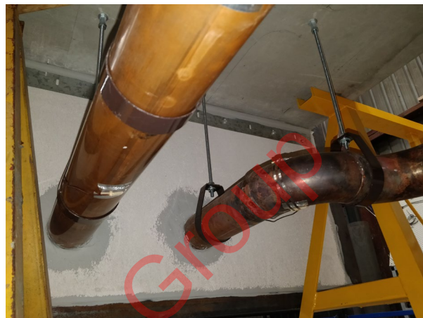
Unwrapped hydrant pipes
